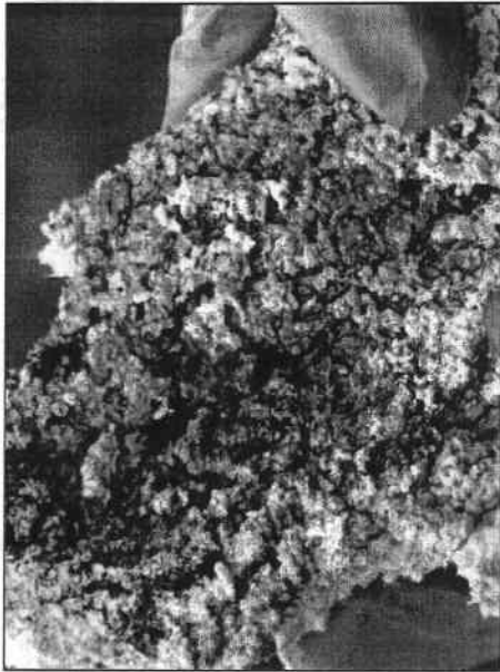
Mold growing on a piece of ceiling tile.
