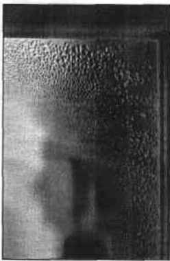
Condensation on the inside of a window pane.
